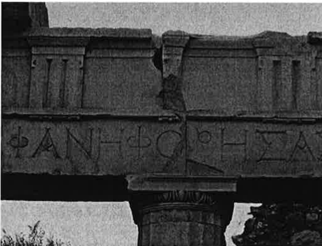
Fig. 17.17. Theatre, logeion . Repair disrupting triglyph.
